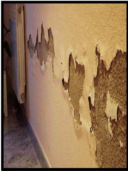
(f) Figure6 Internal view of wall seepage
